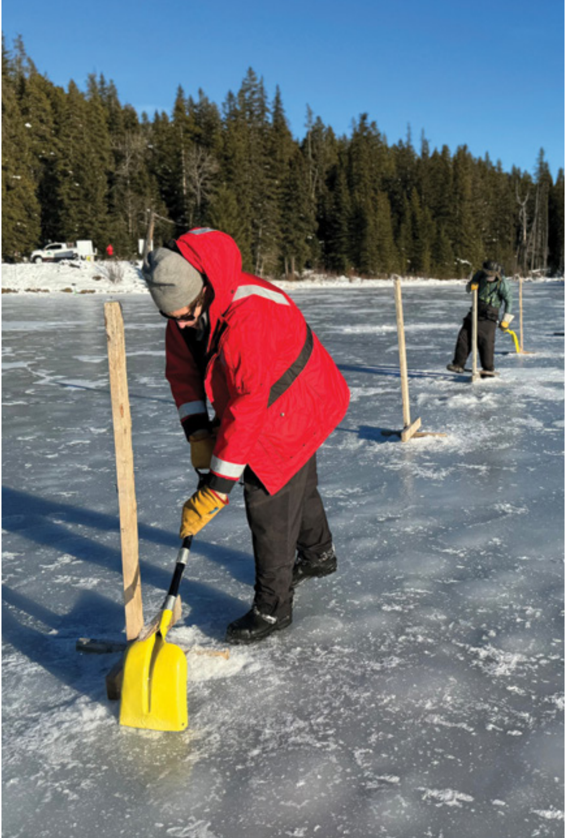
Project: Lake Aeration (Fence installation at Coleman Fish and Game Pond Conservation Site) photo: ACA, Mike Jokinen
