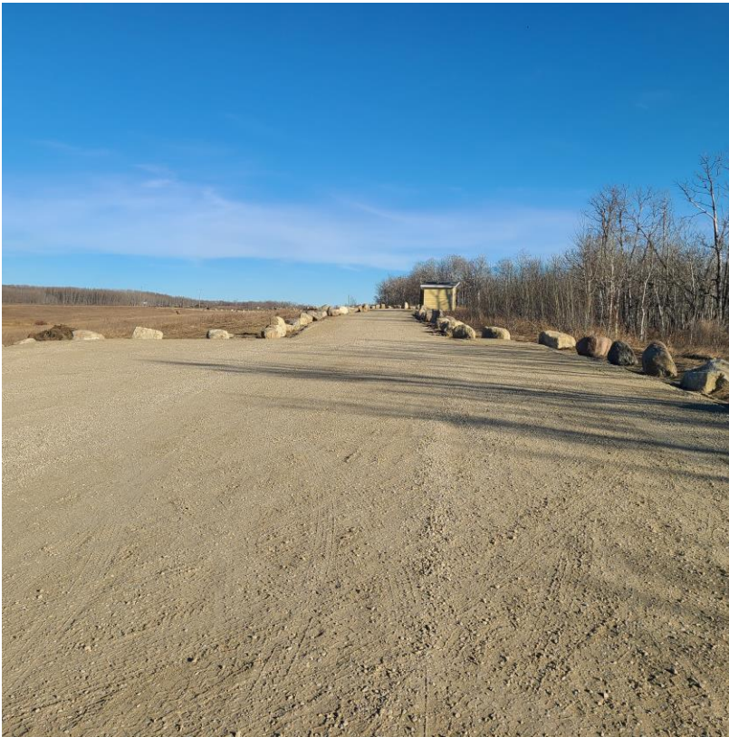
Photo 2. New parking lot and access road constructed at Boulder Lake. Photo: Marco Fontana
