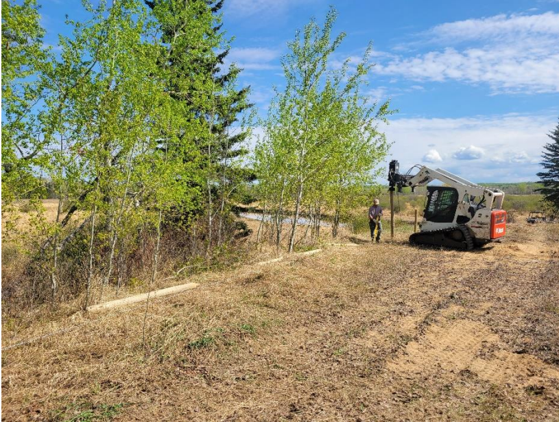
Photo 2. Fence install along the habitat lands on the Owl River for a new RHEA.
