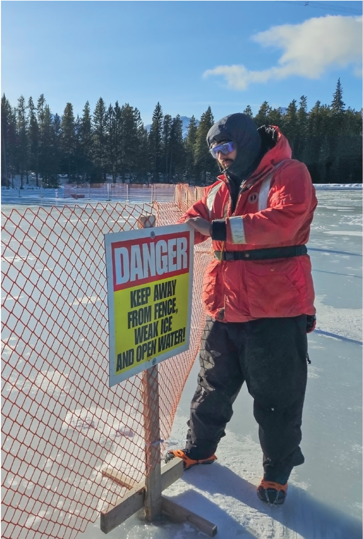
Project: Lake Aeration photo: ACA
