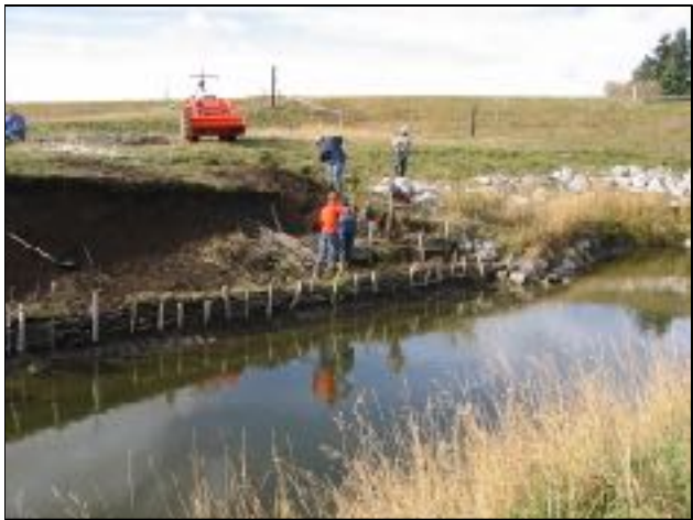
Figure 2. Representatives from the Bearberry Creek Conservation Working Group constructing a bank stabilization project, using bioengineering techniques. (Photo: Chad Judd)
