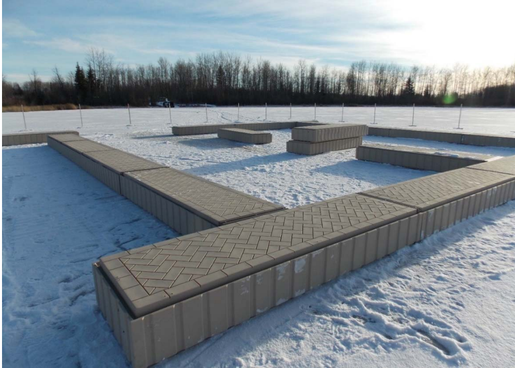
Construction of PolyDock structure for containment of the subsurface diffuser aerator at East Dollar Lake. Photo: Garret Mcken
