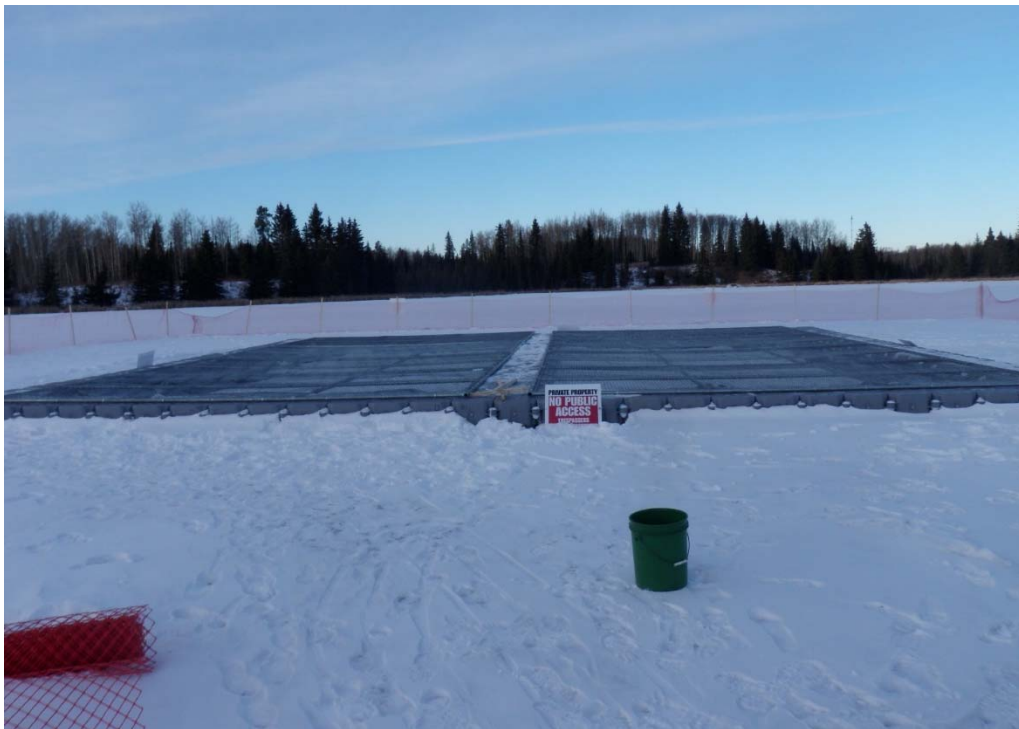
Completed Candock structure with chain-link fencing for containment of the subsurface diffuser aerator at Fiesta Lake. Photo: Kevin Fitzsimmons
