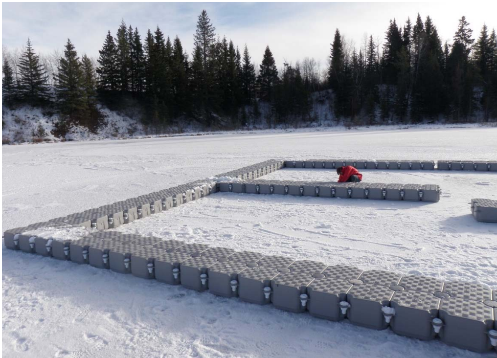
Construction of Candock structure for containment of the subsurface diffuser aerator at Ironside Pond. Photo: Kevin Fitzsimmons
