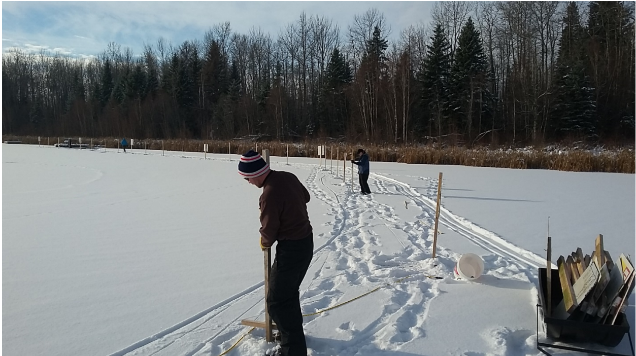
Alberta Conservation Association staff installing perimeter fence at Spring Lake (Stony Plain). Photo: Brendan Ganton
