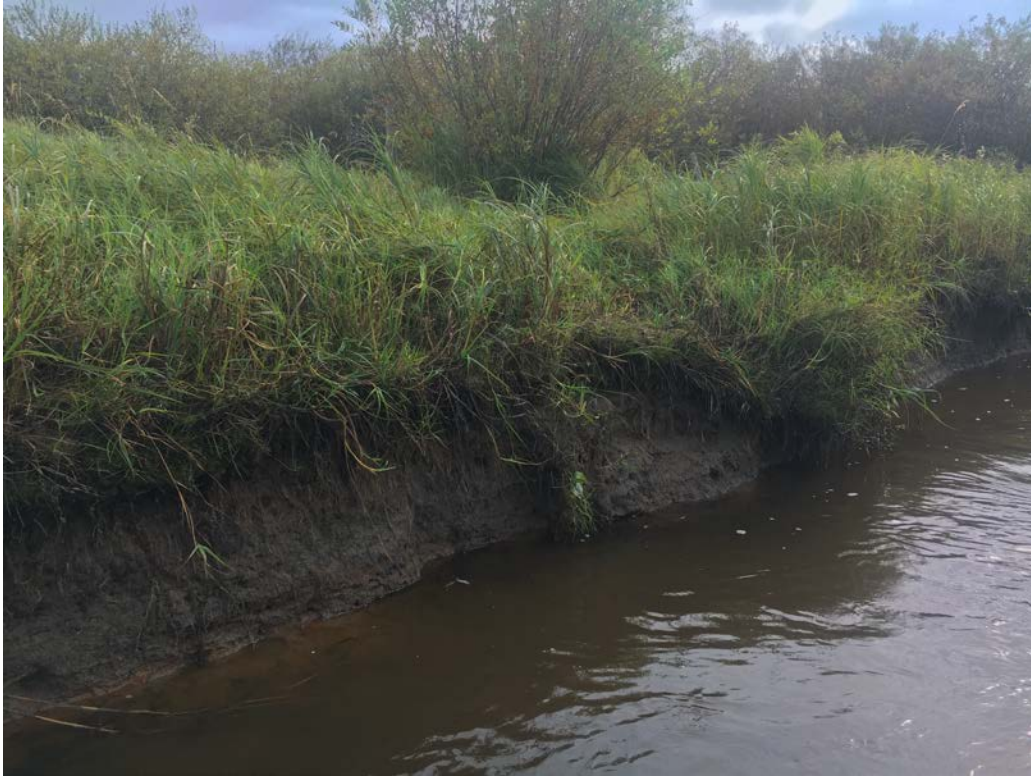
Erosion along the bank of the Owl River following August flooding. Photo: Britt Schmidt
