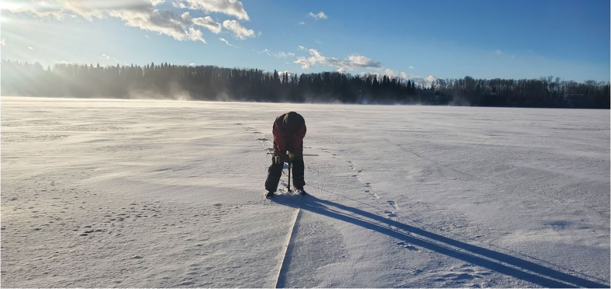
Photo 3. ACA staff drilling safety fence post holes at Millers Lake. Photo: Troy Furukawa
