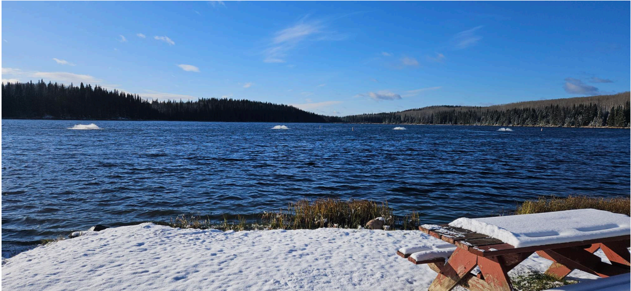
Photo 1. Surface aerators running after installation at Sulphur Lake. Photo: Dave Jackson
