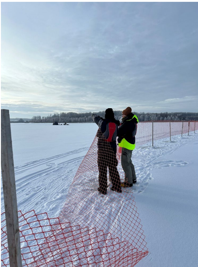
Photo 2. ACA staff members installing safety fence at Hasse Lake. Photo: Ariel Schlereth
