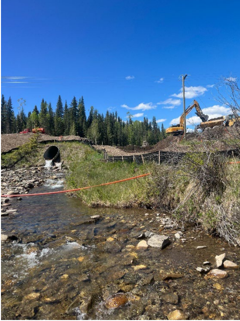
Photo 3. Remediation of the Highway 11 crossing of Gonika Creek west of Nordegg, June 2024. Photo: Isabelle Crawford
