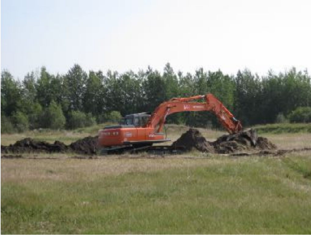
An excavator on North Fawcett 2 Conservation Site creating a “ditch plug”. This activity was identified in the management plan and was a joint project with Ducks Unlimited Canada to restore wetlands on landscapes that have been drained. (Photo: Stefanie van Huystee)
