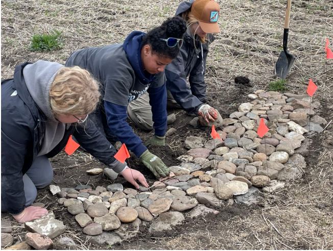
Photo 7. Nature Conservancy of Canada (M. Asante and P. Asplund) and ACA staff members constructing Zeedyk structures to control surface water flow at Manyberries Creek Conservation Site. Photo: Tyler Johns
