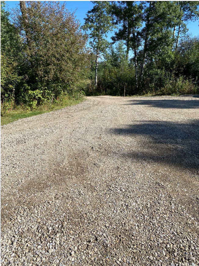
Photo 4. Access road and parking lot improvements completed at Birch Lake. Photo: John Hallett
