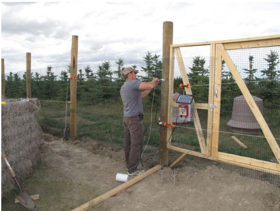
Construction of the large pen used for soft-release trials of pheasants. Photo: Kyle Prince
