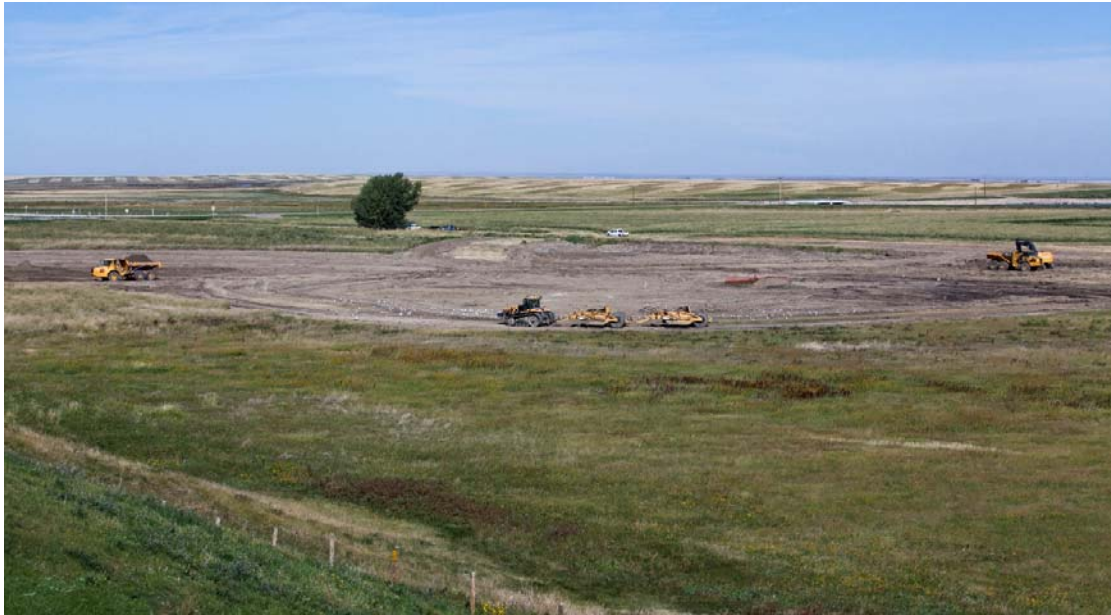
Construction of the wetland on the west end of Ridge Reservoir for the Milk River Ridge Reservoir Water Quality Stewardship Initiative project. Photo: Sam Wirzba
