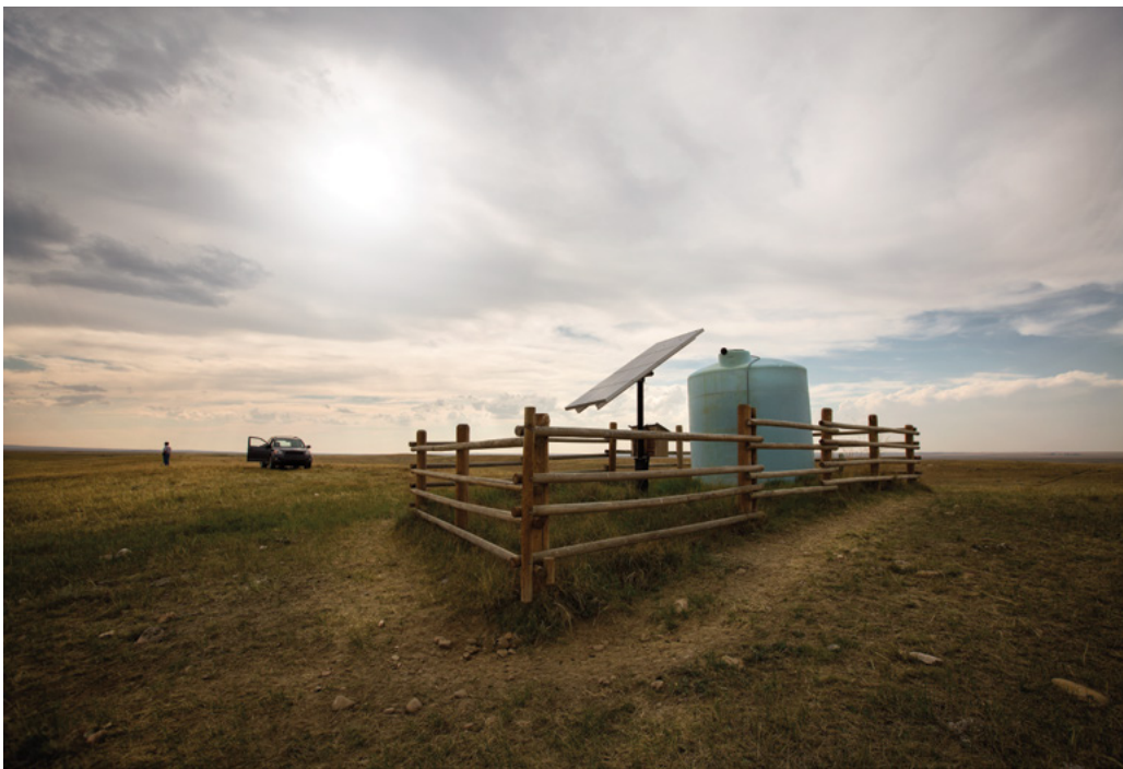
Solar-powered well and trough station.
