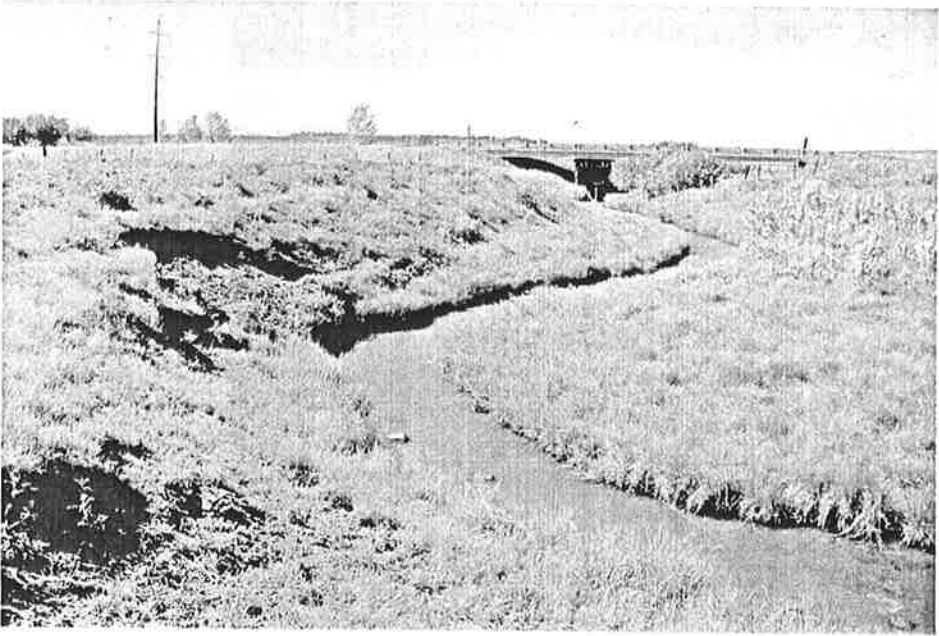
Appendix 6. Beaverdam Creek, site 2 looking downstream at Highway at 568 in the background, July 2003.
